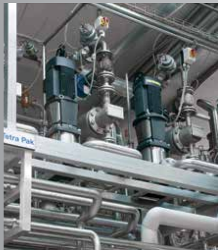
CR pumps installed in a dairy plant
