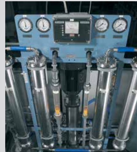
CRN 5 installed in a water treatment plant
